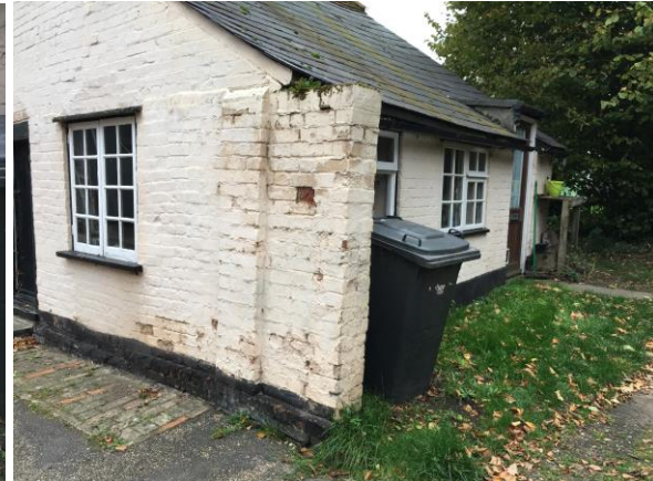
Photograph 8: Protruding wall from 1-6 The Street
